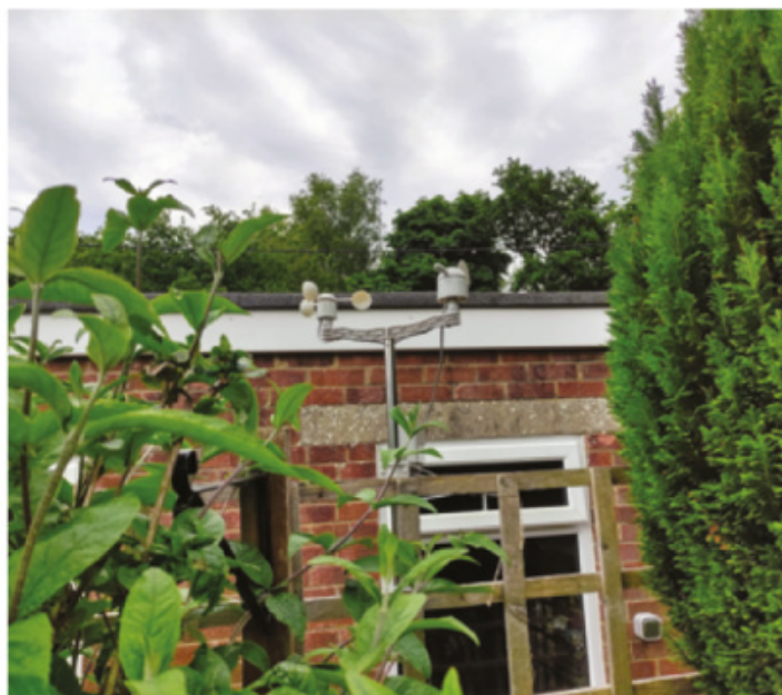
▲ Our weather station's cables go into the garage where a Weather HAT-equipped Raspberry Pi is located – an external weather-proof box would be better, however
